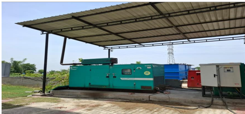
Figure 4.4: DG set at SGC
