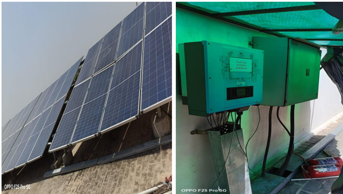
Figure 4.7: Picture showing the installed solar panel
