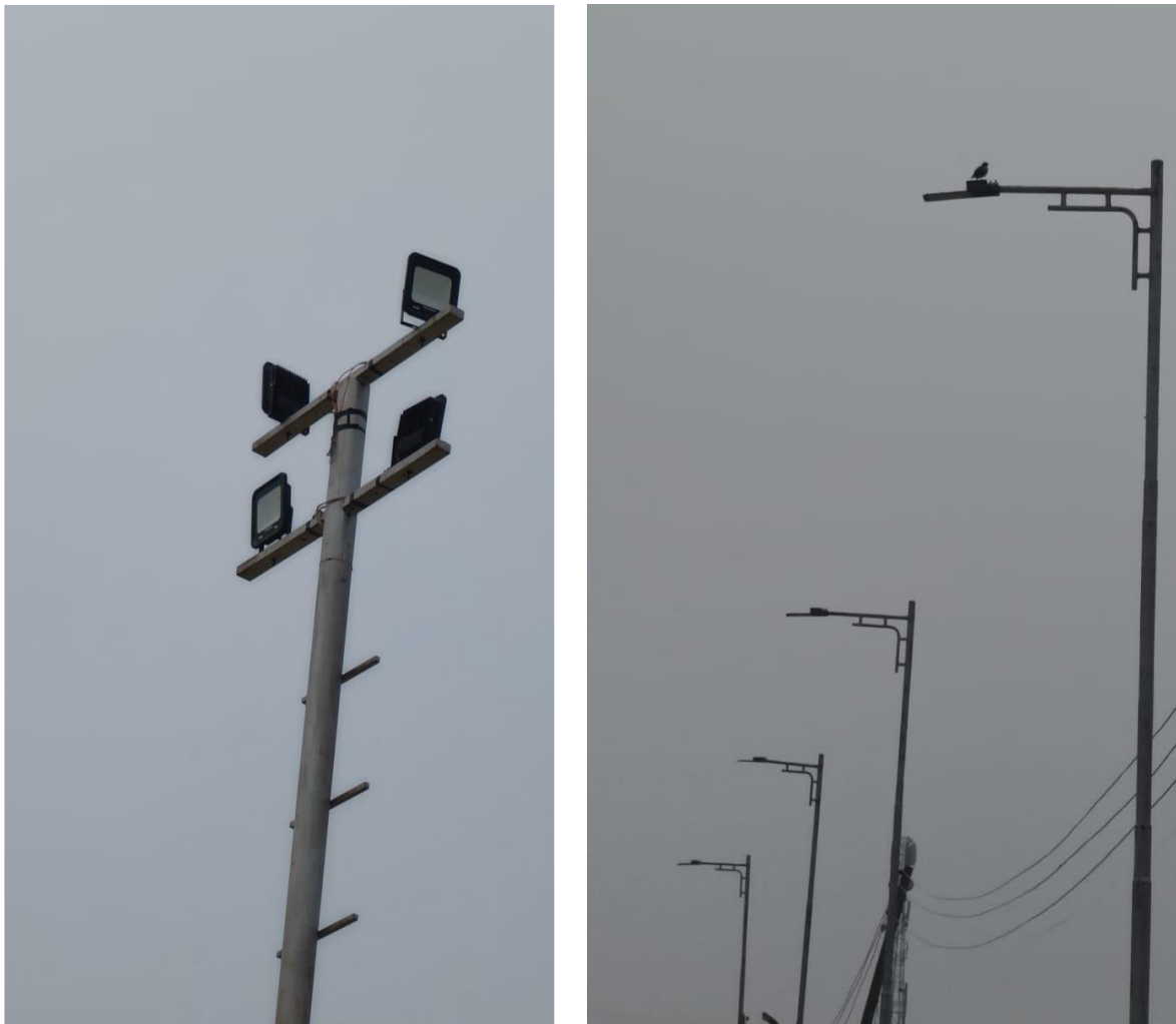
Figure 4-10 Street light used by the college in the campus
