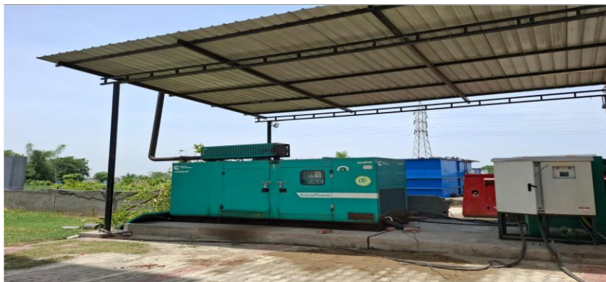
Figure 4-3: DG set at SGC
