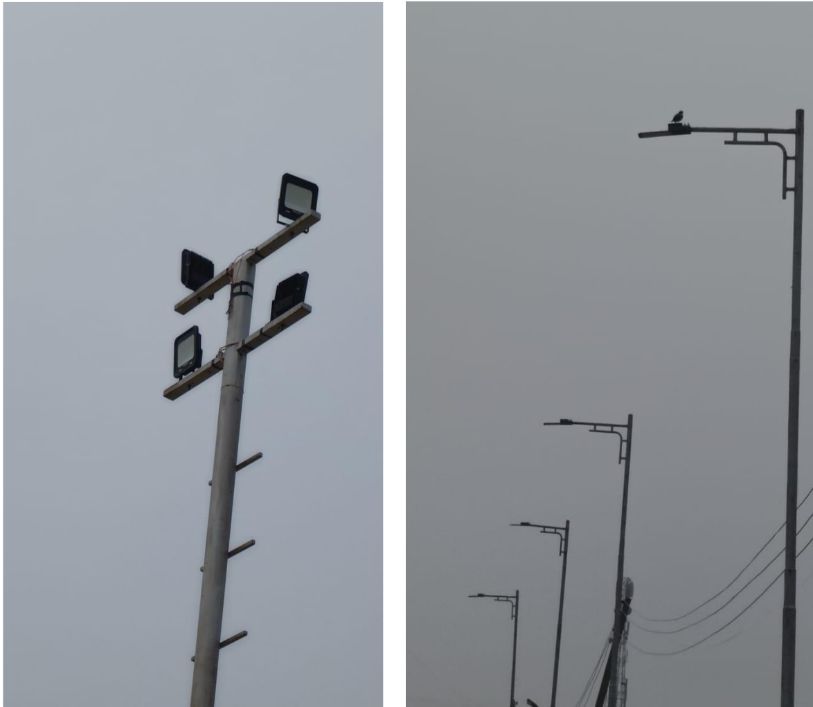
Figure 4-11 Street light used by the college in the campus
